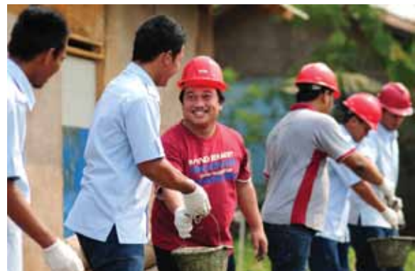
Some houses in Kutamekar Village (Indonesia) only have a dirt floor. Together with the local citizens, Bekaert colleagues helped to build a concrete floor using our Dramix® steel fibers.
