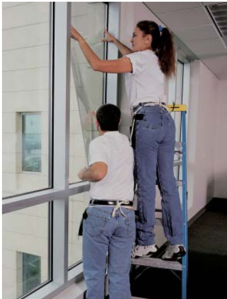
Specialized installers applying window film to keep out the sun's heat and ultraviolet radiation and provide protection in the event of breakage.
